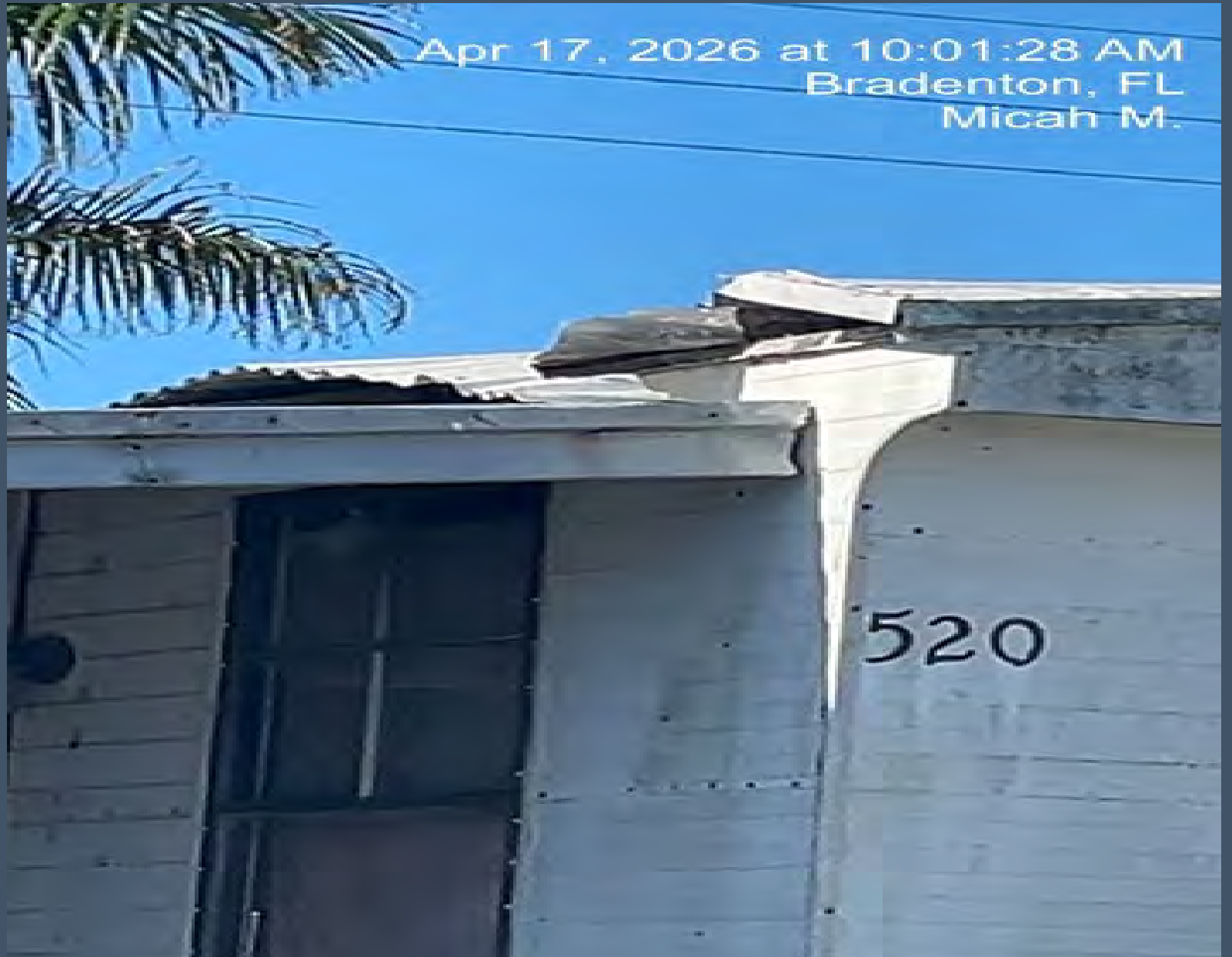
Initial Photo #2 – Damaged Roof
